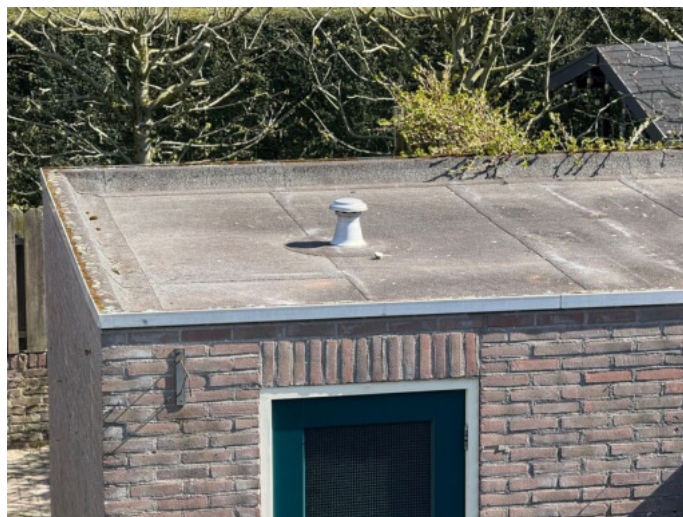
Conditie dak berging
